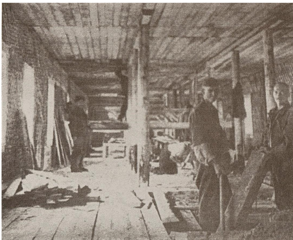
Interior work at the construction of a new barrack in Camp no. 158 in Cherepovets
